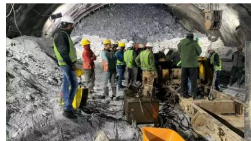
Trapped workers being rescued in Silkyara-Barkot tunnel
